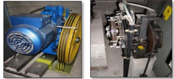
Fig. 2 Modern elevator monitor. Speed controller.
