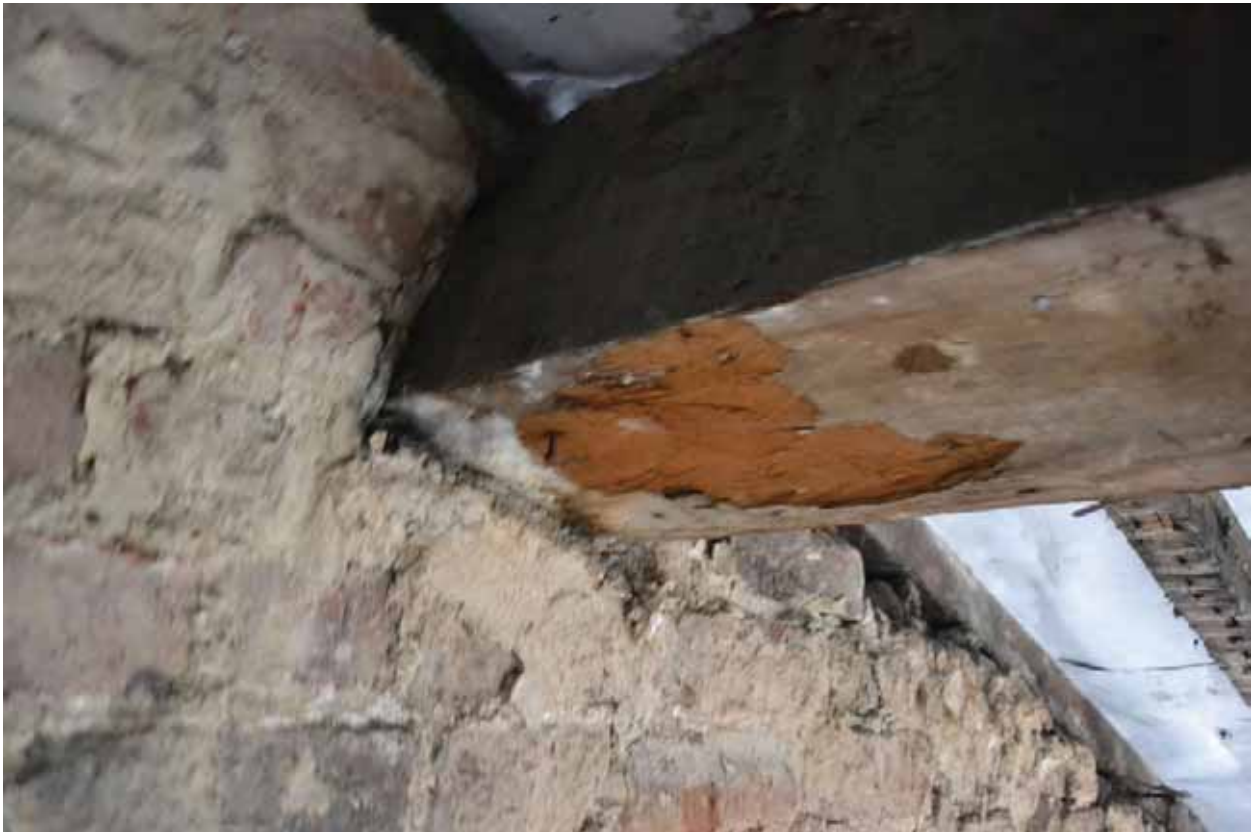
Fig. 129 - Attention needed on the roof timbers in the attic
