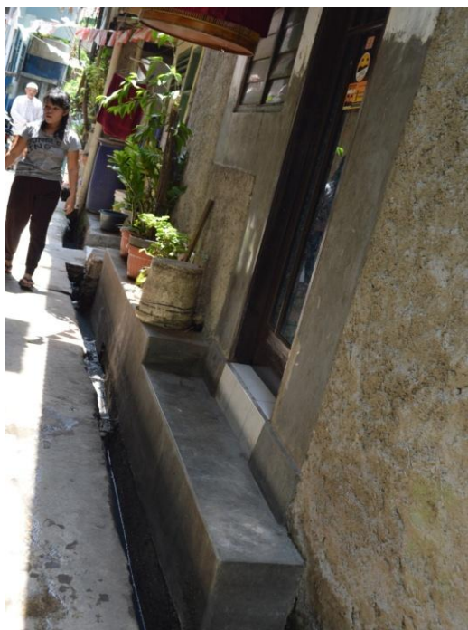
e: Rain water drainage system in Pademngan roads, Jakarta, Indonesia Source: Taken by the researcher in Jakarta, Indonesia, 2013
