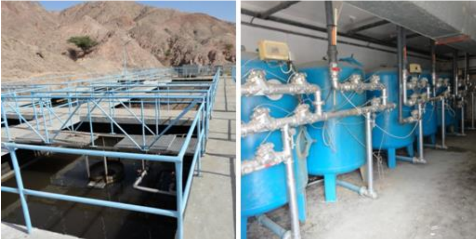
Figure 139 Left: Aeration, Right: Water tanks (Photographed in central water treatment plant shared between Hilton Taba & Nelson Village resort and Movenpick Taba resort by the researcher)
