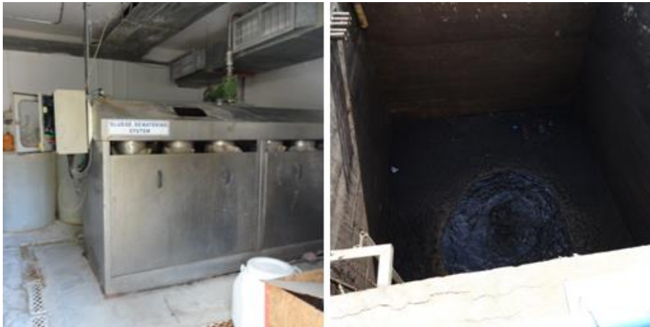
Figure 140 Left: Sludge dewatering system, Right: Final filtration (Photographed in central water treatment plant shared between Hilton Taba & Nelson Village resort and Movenpick Taba resort by the researcher)
