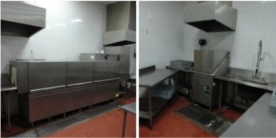
Figure 129 Left: Main dishwasher, Right: Secondary dishwasher (Photographed in Resta grand resort by the researcher)
