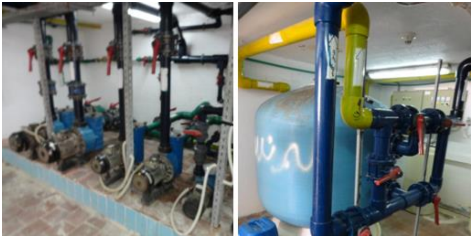
Figure 138 Left: Pumps, Right: Sand filters (Photographed in Hilton Sharm Dreams resort by the researcher)
