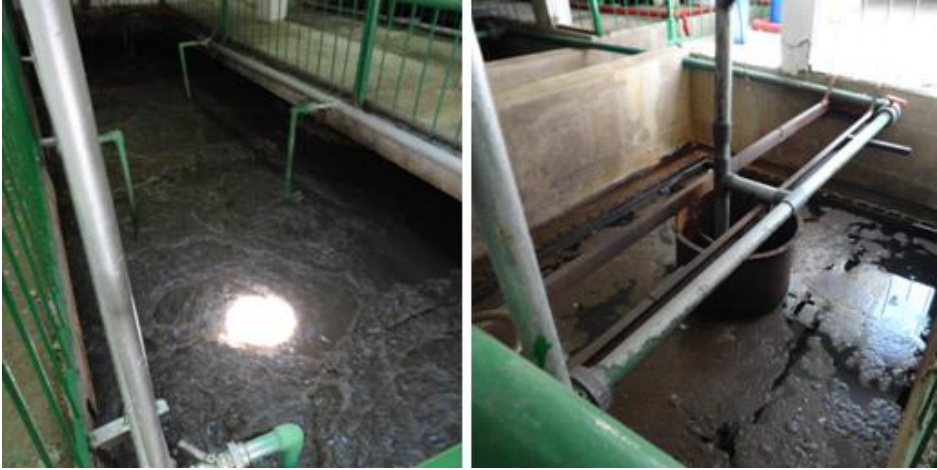
Figure 141 Left: Aeration, Right: Final filtration (Photographed in Hilton Sharm Dreams resort by the researcher)
