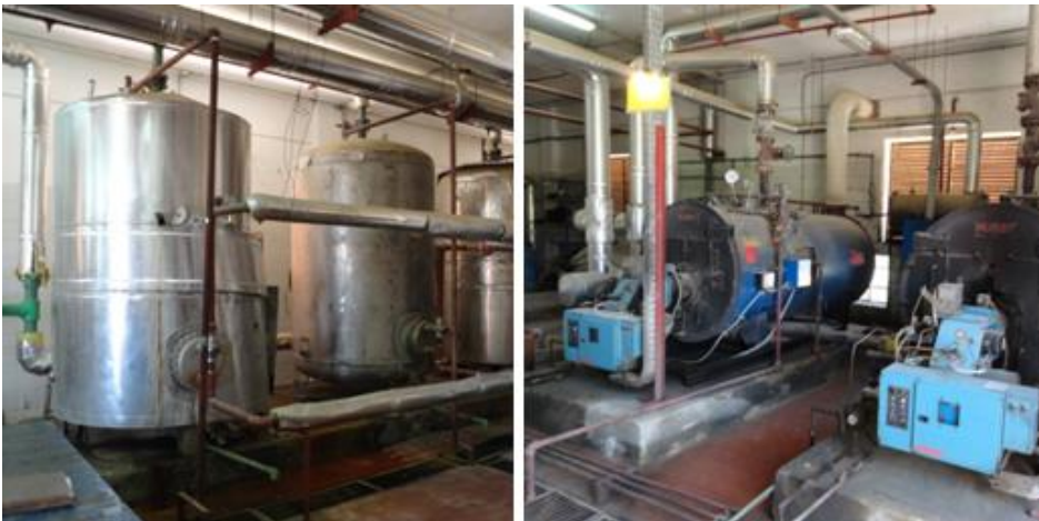
Figure 122 Left: Main boilers, Right: Steam boilers (Photographed in Resta grand resort by the researcher)
