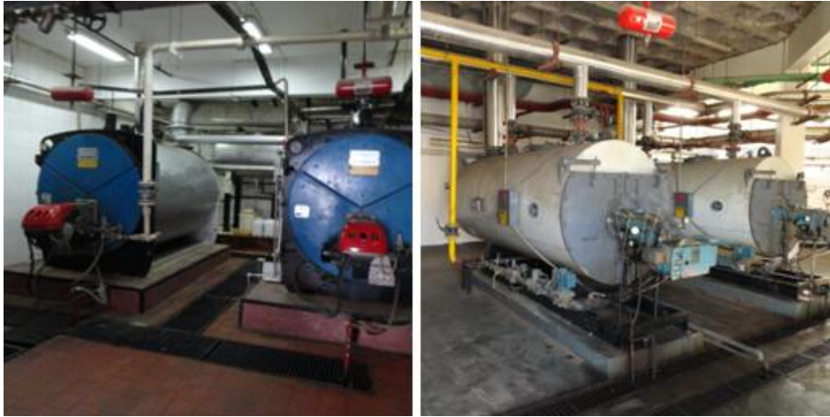
Figure 119 Left: Main boilers (Photographed in Hilton Sharm Dreams resort by the researcher), Right: Main boilers (Photographed in Movenpick Taba resort by the researcher)
