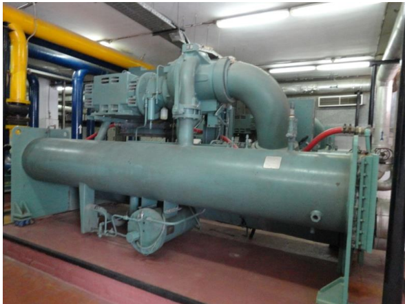
Figure 136 Chiller (Water-cooled system) (Photographed in Hilton Sharm Dreams resort by the researcher)
