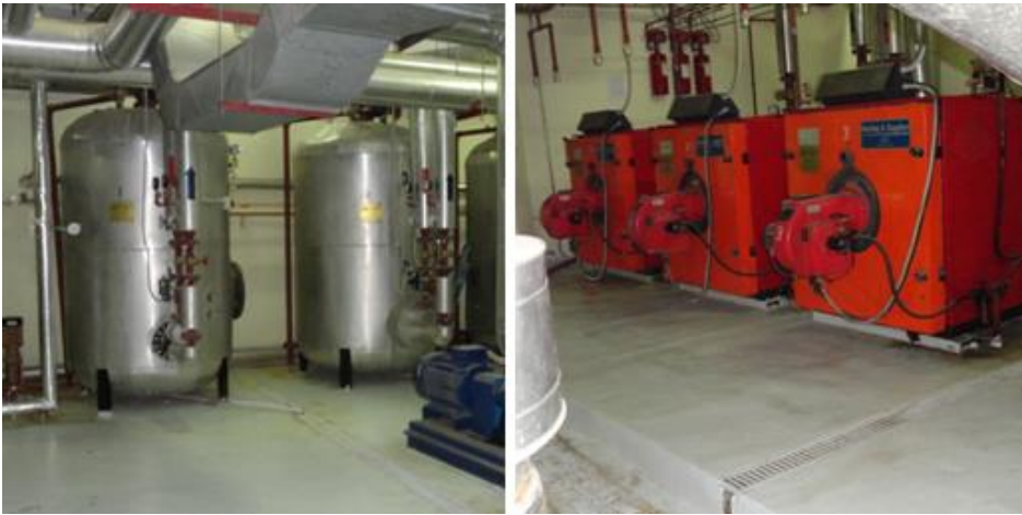
Figure 121 Left: Main boilers, Right: Internal water boilers (Photographed in Hilton Taba & Nelson Village resort by the researcher)
