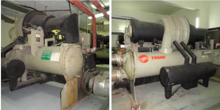
Figure 135 Left: Chiller (Water-cooled system) (Photographed in Hilton Taba & Nelson Village resort by the researcher), Right: Chiller (Water-cooled system) (Photographed in Movenpick Taba resort by the researcher)
