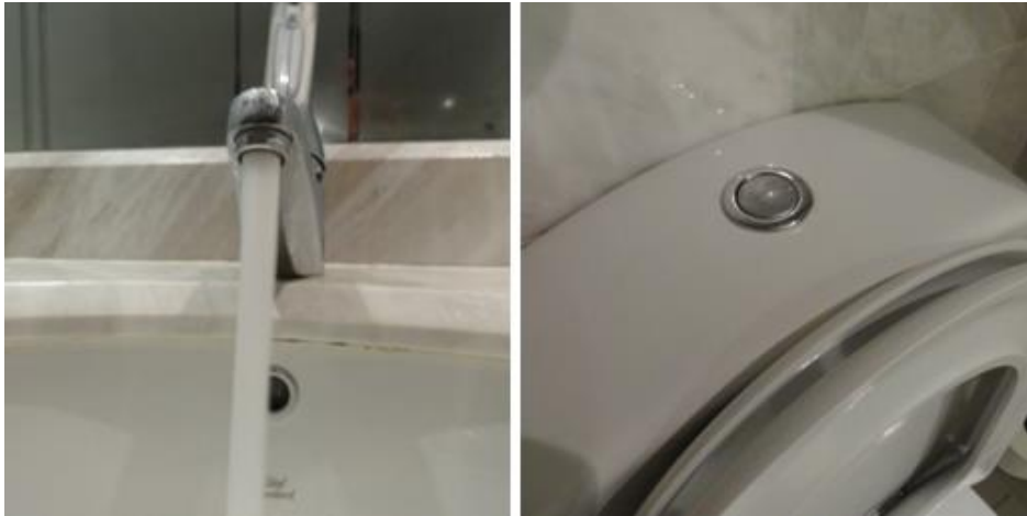
Figure 123 Left: Taps (aerators used), Right: toilets (single flush) (Photographed in Hilton Taba & Nelson Village resort by the researcher)
