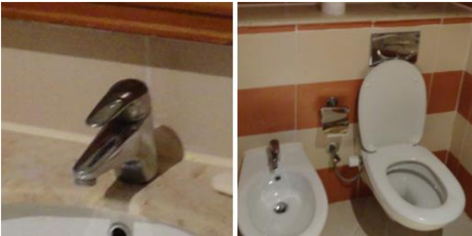
Figure 126 Left: Taps (aerators used), Right: Bidets and toilets (dual-flush) (Photographed in Resta grand resort by the researcher)
