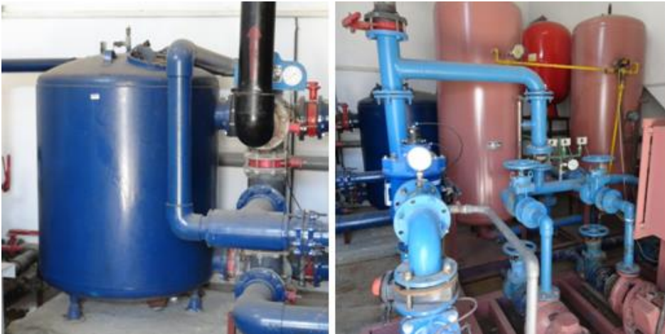
Figure 142 Left: Sand filters, Right: Irrigation pumps (Photographed in Movenpick Naama Bay resort by the researcher)
