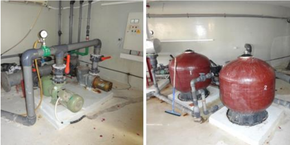
Figure 137 Left: Pumps, Right: Sand filters (Photographed in Hilton Taba & Nelson Village resort by the researcher)
