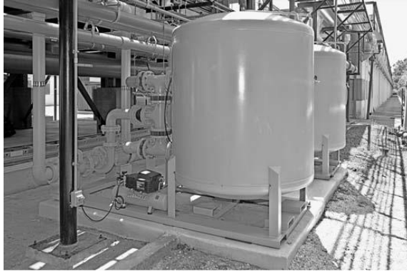
Figure 69 Sand filters used to remove residual biological flocs and precipitates following pretreatment of treated feed-water for a cooling water system (Asano, Burton, Leverenz, Tsuchihashi, & Tchobanoglous, 2007)
