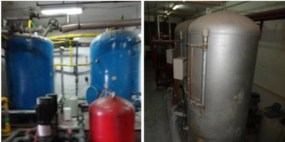
Figure 118 Left: Water tanks (Photographed in Hilton Sharm Dreams resort by the researcher), Right: Domestic water tanks (Photographed in Movenpick Taba resort by the researcher)
