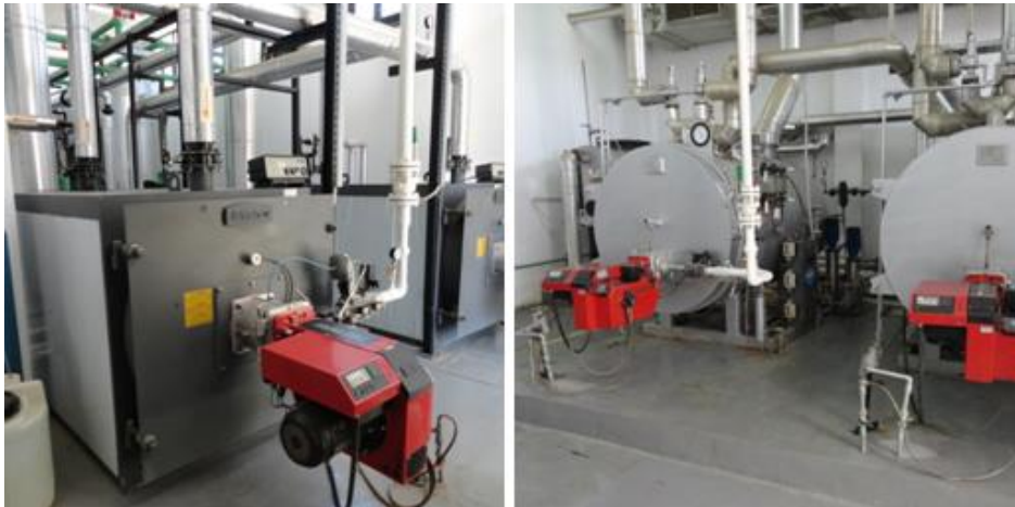
Figure 120 Left: Main boilers, Right: Steam boilers (Photographed in Movenpick Naama Bay resort by the researcher)
