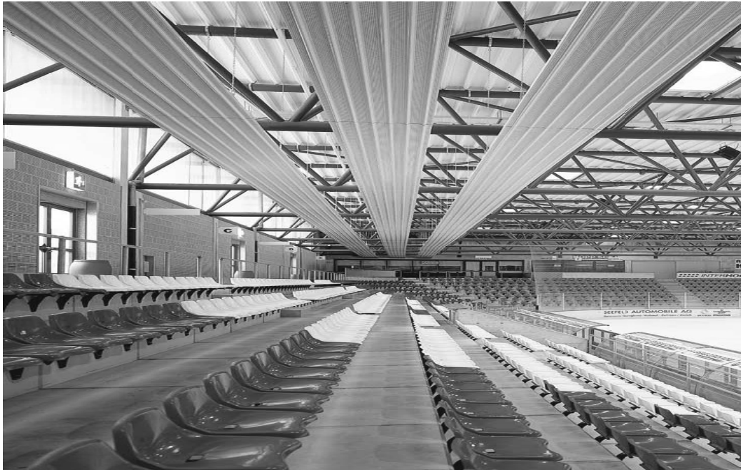
Figure 2- radiant panel cooling system in an open sport hall 45
