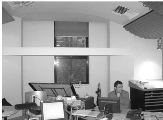
Figure 5- Chilled beam as detailed in prototype office 13
