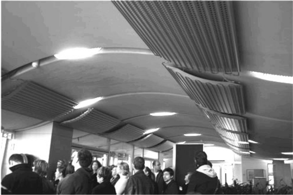
Figure 5- Interior view: Radiant ceiling panel 11
