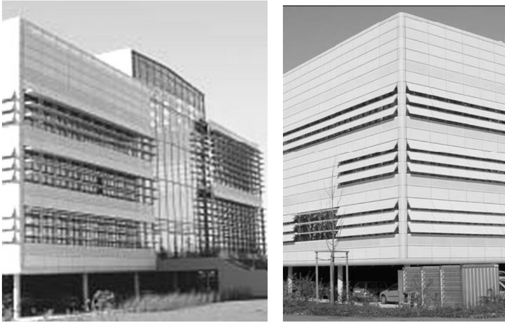
Figure 4- Application of Fabric membrane stretch shading louvers onto the building glass façade, Baader Bank, Germany 26
