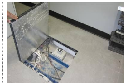
Figure 4.16: Cables Distribution system.
