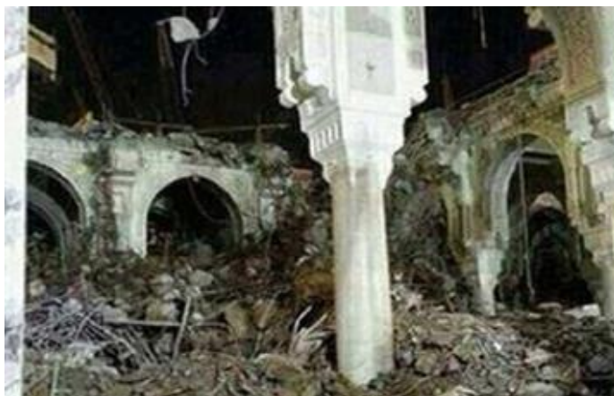
Figure (2-5): A Partial collapse in the Haram Expansion Building during Construction
