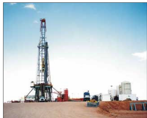
Fig.9-25. Drilling water wells in the desert is a crucial element for agriculture activities
