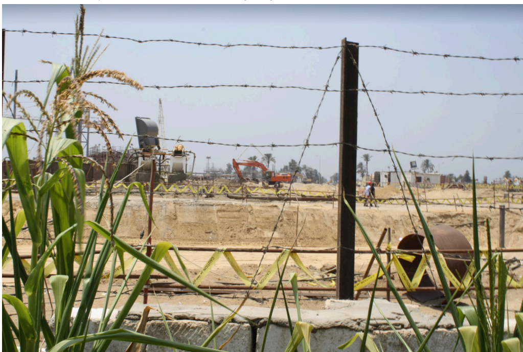
Construction takes place on the World Bank-financed North Giza Power Project Original image by Bank Information Center
