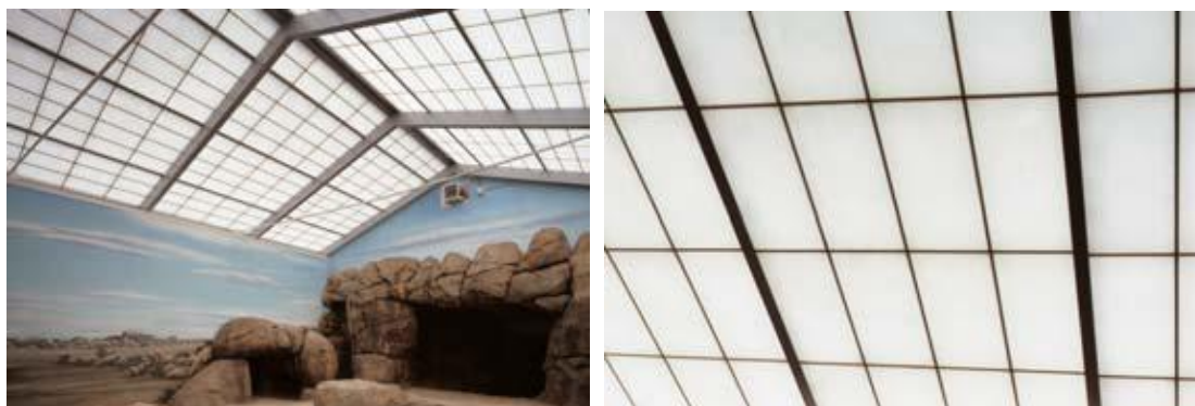
Figure 3.59 Insulated roof by using nano gel at County Zoo, Milwaukee, WI. USA.
