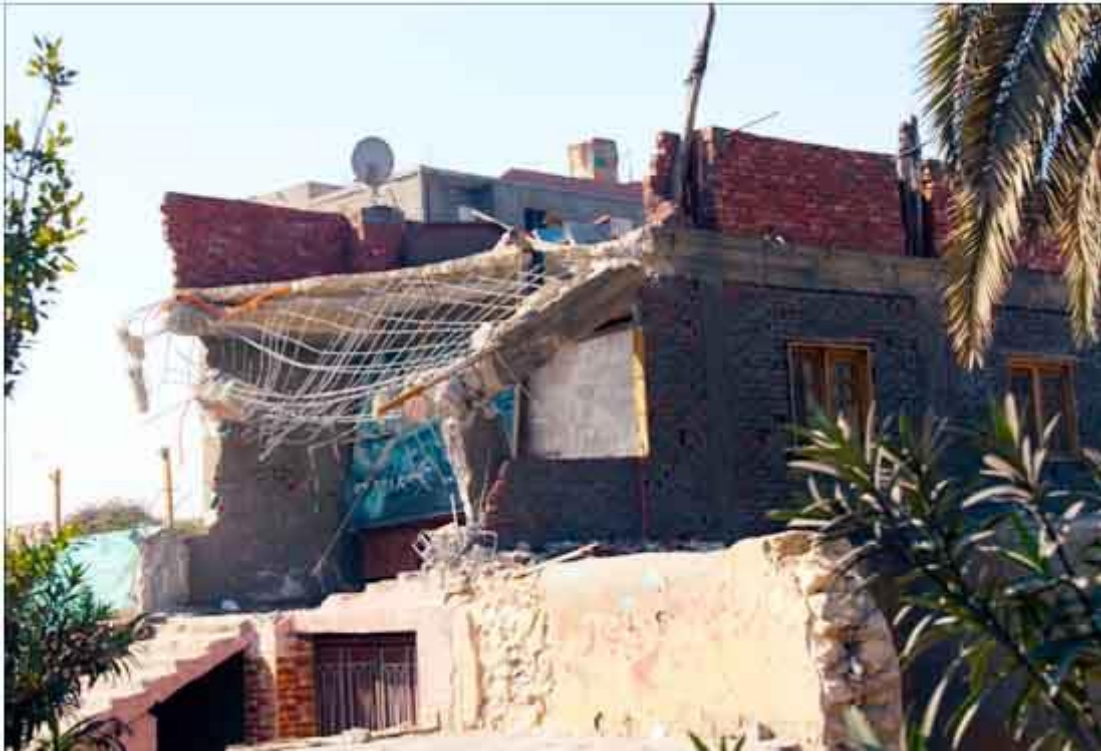
Above: Fig.(42), Photo is taken by researcher. It shows the steps that people follow when violating the law. They managed to build a stair case, that rises over the present wall, to make an entrance on the main road (Nasr st.). Then the rest of the building is constructed inside the cemeteries inside one of the existing hawshes. Date taken: 08/11/2014 - 12:10 PM.
