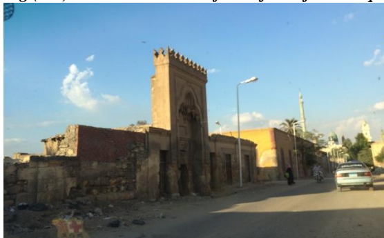
Fig.(164): Deteriorated front of a historical mausoleum
