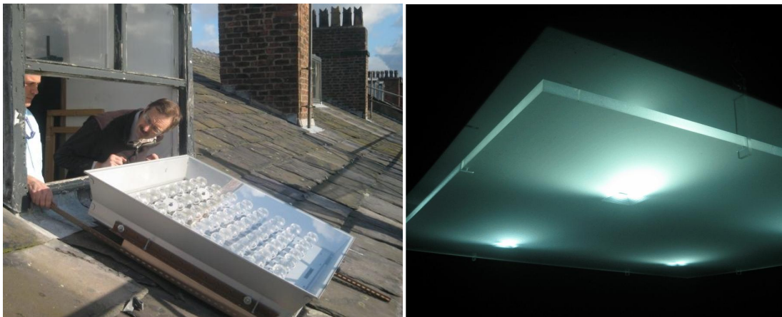
Figure 7.1: Parans solar panel installation in the Uni. Of Livrepool (left); Figure 7.2: Parans 'L1-large' luminaire (right).
