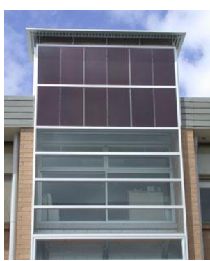
Figure 2. 54 Solar Panels in the elevation. . “www.worldarchitecturenews.com”.
