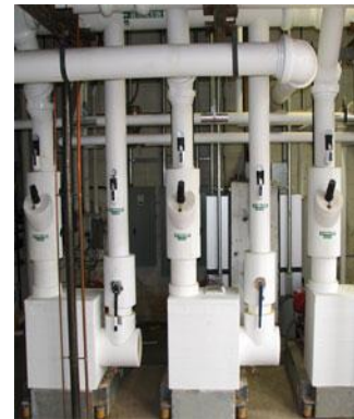
Figure 2. 57 pipes for HVAC system. “www.worldarchitecturenews.com”.
