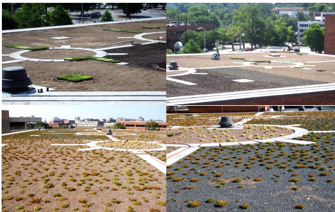
Figure 4.24 Top : Construction phase for installing a pilot vegetative roof on top of Hulsey Center.
