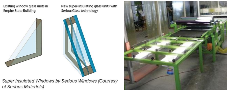
Figure 4.51 Left: New windows installed in the Empire State building. Right: The temporary window refurbishing production line at Empire State Building Source: Harrington, E., and Carmichael, C., (2009), Project Case Study: Empire State Building, Rocky Mountain Institute Report, Via URL: http://www.rmi.org/Content/Files/ESBCaseStudy.pdf , accessed June 9, 2013.
