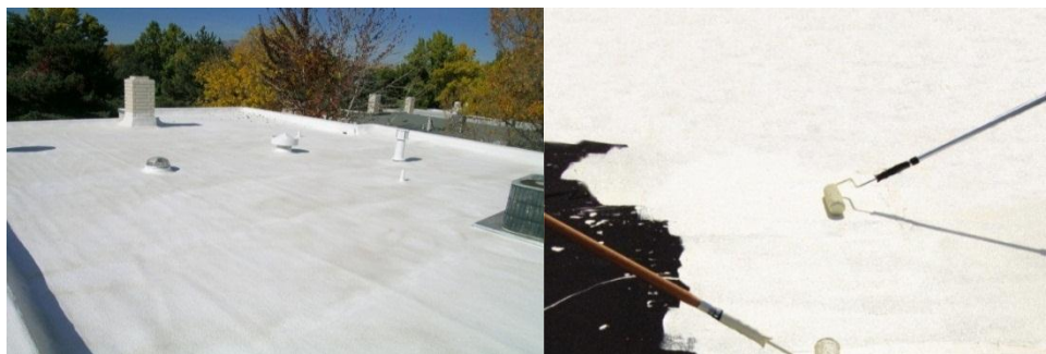
Figure 4.26 Cool Roof (Reflective white colored)
