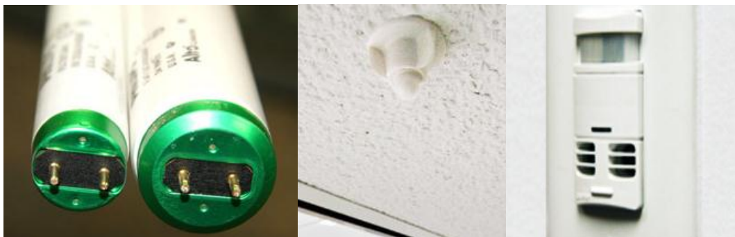
Figure 4.34 Left: The T-8 lamps and high efficiency electronic ballasts that were installed Middle: photocell that detects natural light. Right: Occupancy sensor.
