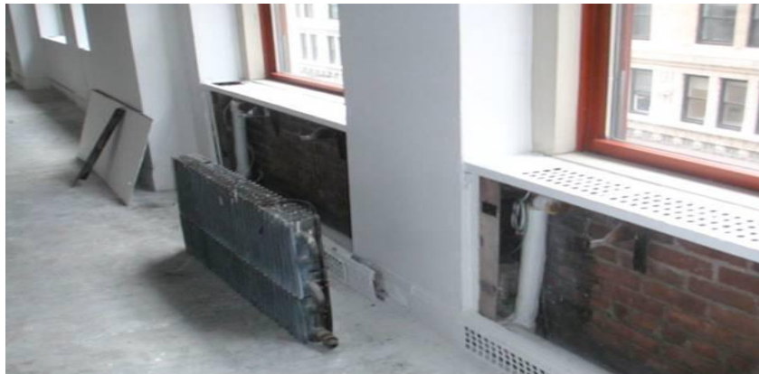
Figure 4.52 Radiative barrier installed in the Empire State building.
