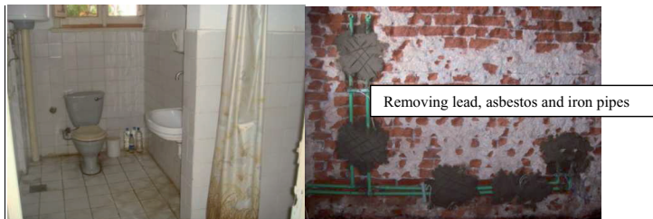
Figure (5.26) Existing bathroom & Poly polypropylene pipes in water supply system in the villa bathrooms (Taken by the researcher, 2010)
