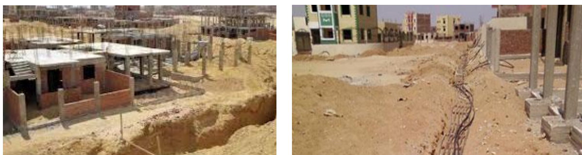
Figure 1. "Build your Home, Ibni Baetak ", 6 October New City, Egypt – delayed implementation of the "Public Product": infrastructure networks and external spaces.
