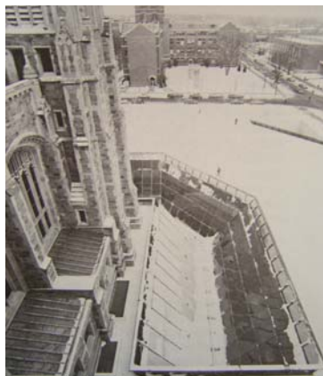
Fig (3-46): The sloping skylight viewed from the roof of the original building
