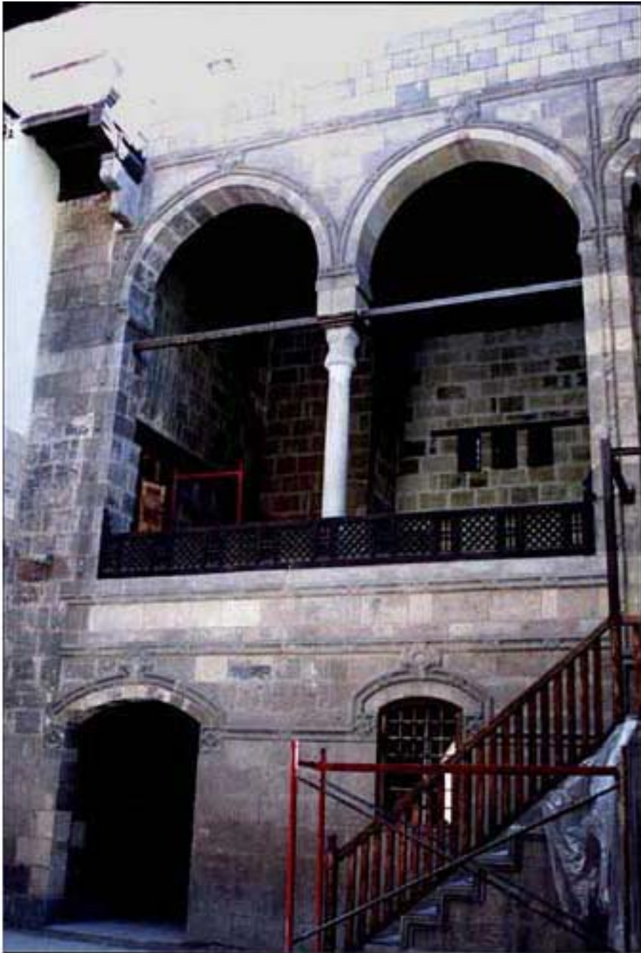
Figure 4: The 2-bay Maq'ad of Zaynab Khatun, Ottoman Phase This Maq'ad is a very typical Ottoman one in its form. Photo by Arch. A. Hassaballah
