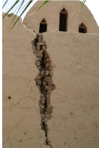
Figure 3: The cracks in a house wall, Qurna village- Hassan Fathi - Luxor – Egypt, Taken by the Author
