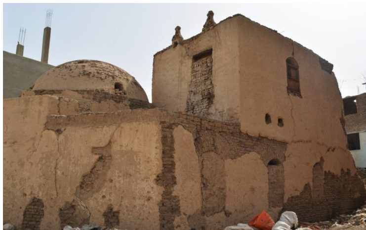
Figure 8: Wall Bulging and Slumping, El.Qurna- Luxor, Egypt, Taken by Author
