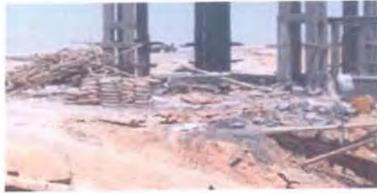
Fig. (7-54) Construction waste mixed with cement sacs
