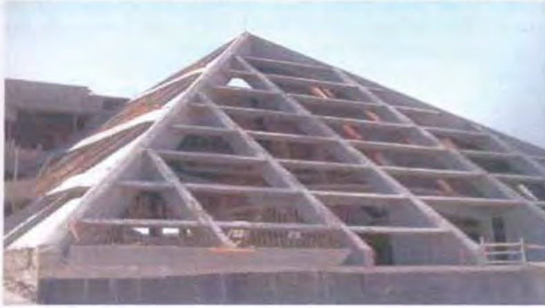
Fig. (7-14) The main building atrium under construction The RHS illustrates the first sandwich layer before the heat insulation was placed.
