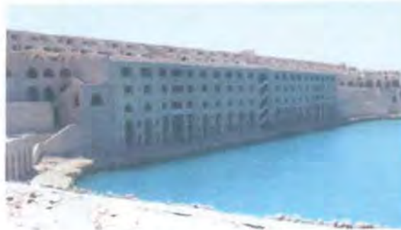
Fig. (7-37) A general view for the guest rooms under construction over viewing the in-land manmade lake
