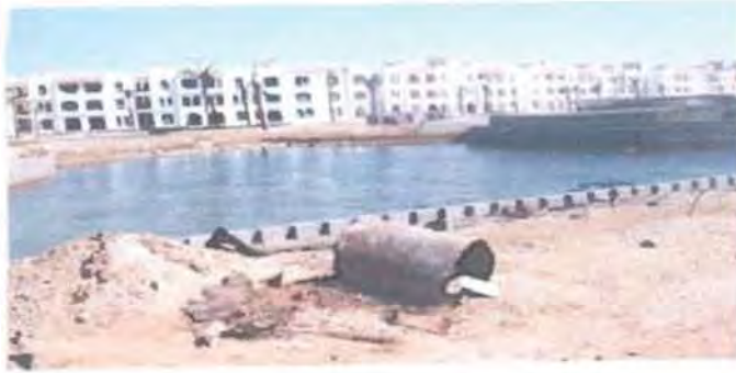
Fig. (7-71) Improper construction waste handling
