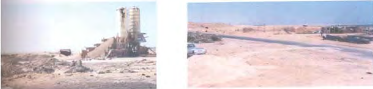
Fig. (7-51) Concrete batch plant Fig. (7-52) Steel bars workshop & waste shuttering wood collection
