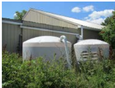
Fig. 2 A side view of the Horticulture Services Building (Macdonald Campus, Sainte-Anne-de-Bellevue, QC, Canada) (Adamowski, 2014)
