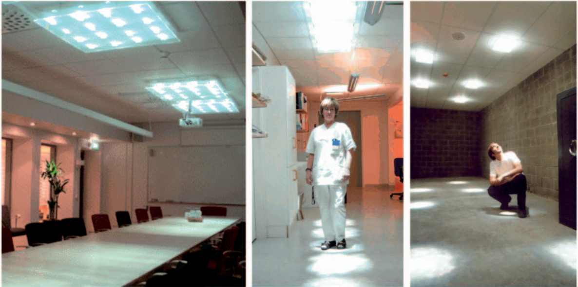
Figure 13 Daylight-only luminaire in use (from Reference 4)
