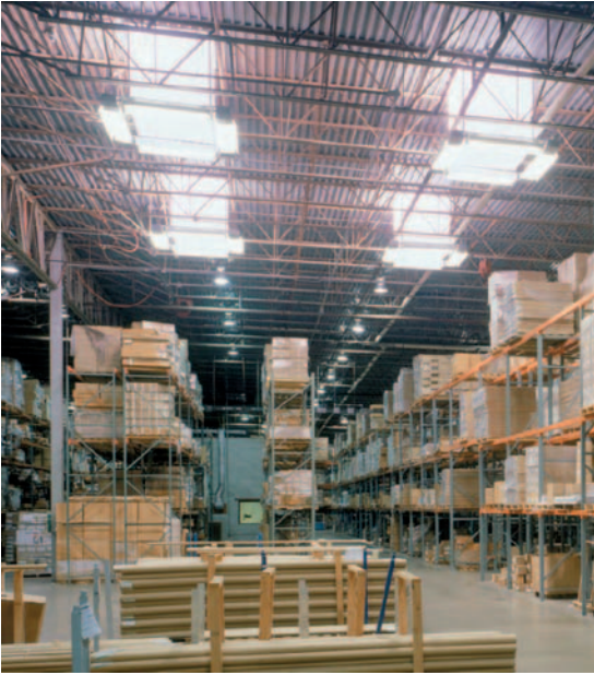
Figure 4 Integrated skylight luminaires (ISL) in a warehouse
