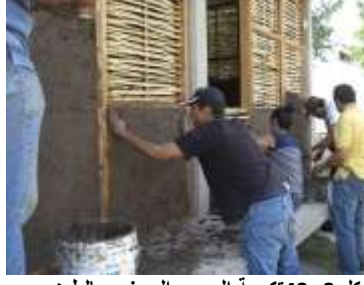
شكل 3- 43 تكسية البوص العرضي بالطين المعجون بالقش بمبنى الاجتماعات المصدر: Pedro Bravo, 'In 4 Days, 100 Volunteers Used Mud and Reeds To Build This Community Center in Mexico', in Archdaily < http://www.archdaily.com/628163/in-4-days-100-volunteers-used-mud-and-reeds-to-build-this-community-center-in-mexico > [accessed 12 October 2015]
