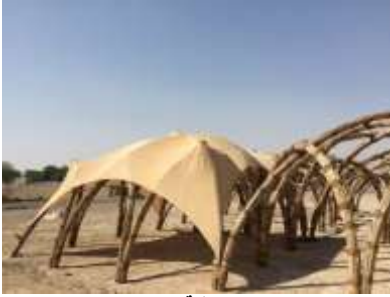
شكل 3- 68 تركيب التغطية من الكتان المصدر: Peter Shehan, 'Palm Leaves Food Shelter', in Design Boom News Letter < http://www.designboom.com/architecture/sandra-piesik-3-ideas-ltd-food-shelter-the-sabla-al-ain-unesco-03-27-2015/ > [accessed 22 September 2015]
