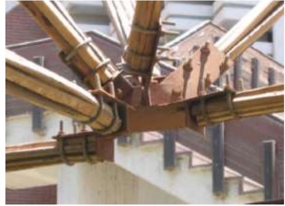
شكل 5- 40 وصلة حرف ال U لضم العناصر الإنشائية المصدر: Raga, Tamer, 'USE OF PALM MIDRIBS AS STRUCTURAL ELEMENTS' (MSc Thesis, Ain Shams University, Department of Engineering, 2010), p. 60.
