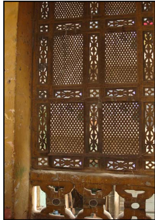
Figure 3-40 Wooden Screen on a 19 th century house - Harit al-Fu'ād in Sayida Zaynab
