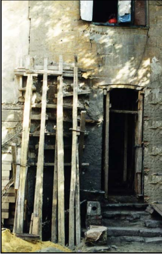
Figure 5-19 Support for a bulging façade for partial reconstruction in Bayt Sitt Sabah
