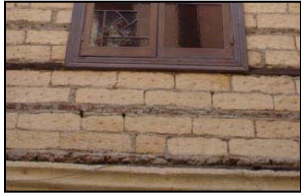
Figure 5-8 Wooden stitching on the sill of the window
