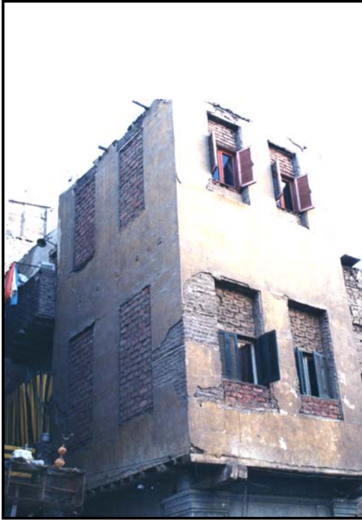
Figure 4-56 Overview of Bayt Abu al-Rūs seen from al-Mahgar Street before intervention (January 2005)
