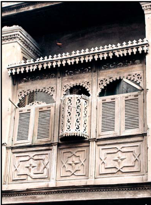
Figure 3-34 Mashrabiyya of Bayt al-Ghandūr, shutters with upper hinges and water jar booth.
