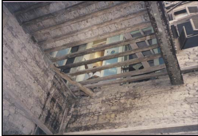
Figure 4-8 Bayt Sukkar: Rehabilitation in progress for the wooden beams and floor layers of the reception area in the first floor (August 1998)
