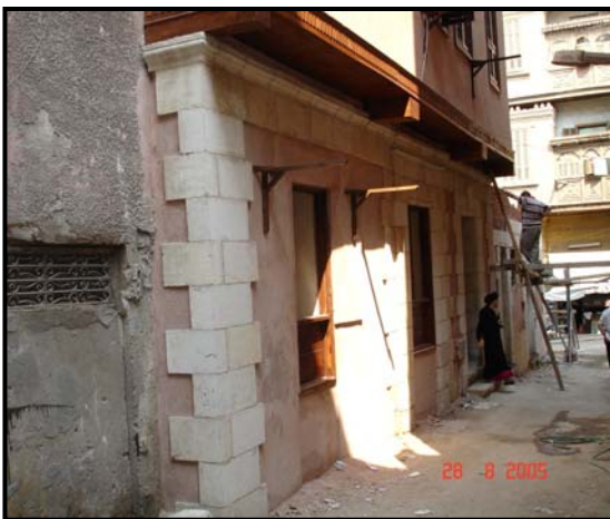
Figure 4-105 The ground floor facade after intervention (August 2005)
