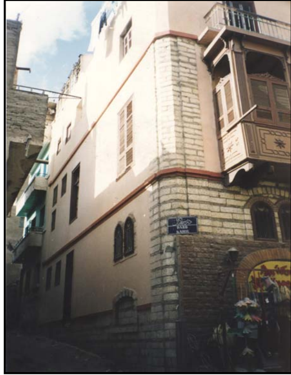
Figure 4-15 The façade of Darb Kaḥīl after rehabilitation of the lower 1.2m stone newly built replacing the old decayed walls (December 1998)
