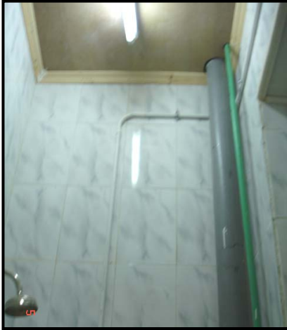
Figure 4-78 New PVC pipes for the sewage system and new Poly propylene pipes for the water supply system, September 2005.
