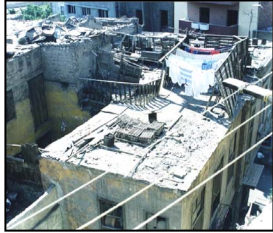
Figure 4-25 Bayt Al-Sitt 'Awaṭif, the condition of the roof before intervention (December 1998)
