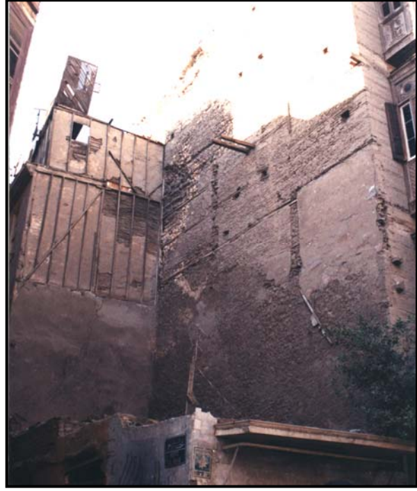
Figure 4-83 The southern wall before intervention (April 2005)
