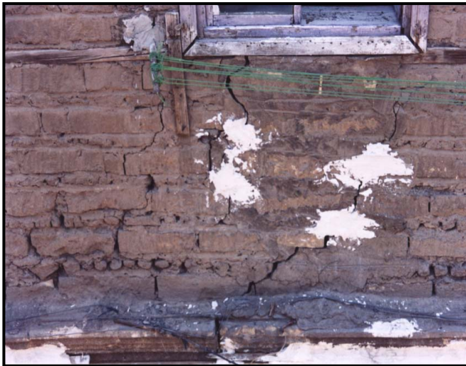
Figure 4-51 Façade cracks - before intervention (May 2004)
