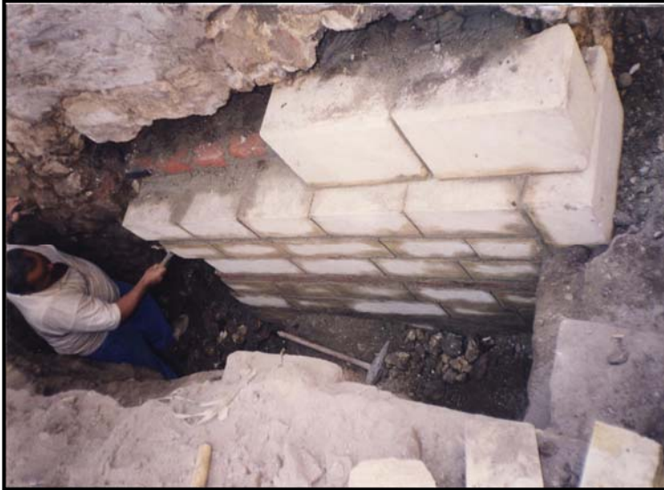
Figure 5-17 damaged foundation walls being replaced from the ground level up. East wall of Bayt al-Sitt 'Awatif during rehabilitation (December 1998)
