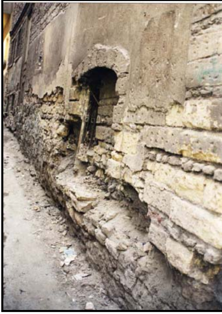
Figure 5-10 Decayed wall of Bayt Sukkar before rehabilitation (1997)
