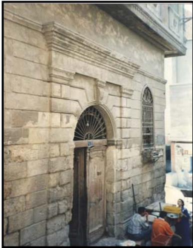
Figure 4-29 Entrance portal before rehabilitation. North façade of Bayt Al-Sitt 'Awaṭif overlooking Ḥarīt Wikalit Al-Sham' (June 1998)
