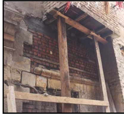
Figure 4-60 Rebuilding the deteriorated section of the masonry wall beneath the balcony of the first floor (Before intervention), October 2004.
