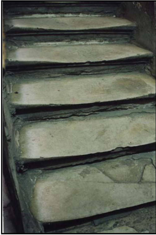
Figure 5-20 Decayed stone steps of Bayt Sukkar
