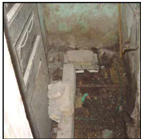
Figure 4-79 dilapidated condition of the ground floor toilet, February 2005.
