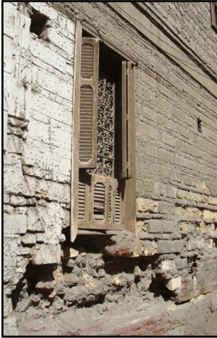
Figure 5-11 Typical decay of walls close to street level
