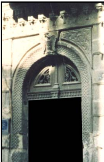
Figure 3-47 Doorway at sikkit al-Kūmi Street with stone carving ferforgée and wood carving
