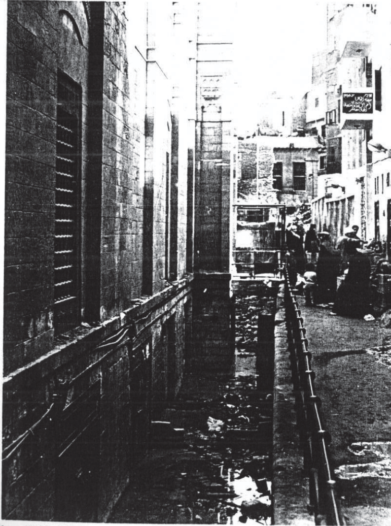
Fig. (21): Mosque of Al-Saleh Talai, The entrance, the height to which water is drawn into the stone by capillary action.
