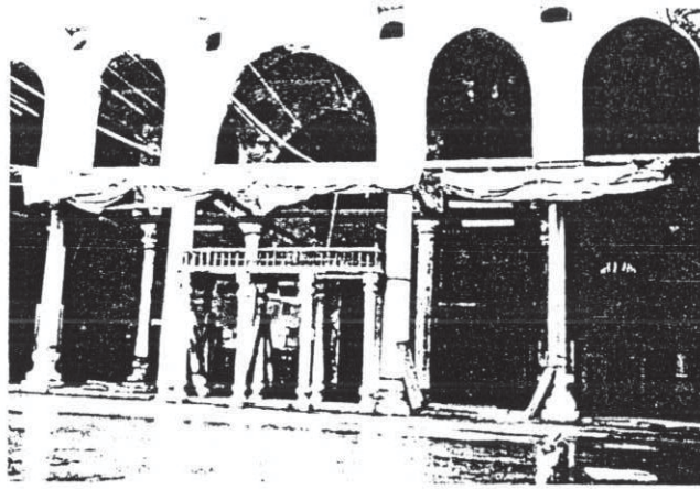
Fig. (20)*: Mosque of Al-Saleh Talai, Cairo, Water Lying more or less permanently above the stone paving of the courtyard.
