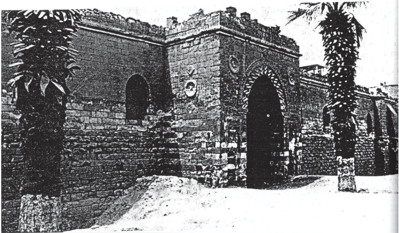
Fig. (22)*: Mosque of Baybars, Ground water drawn upward by capillary attraction destroying the stone work.
