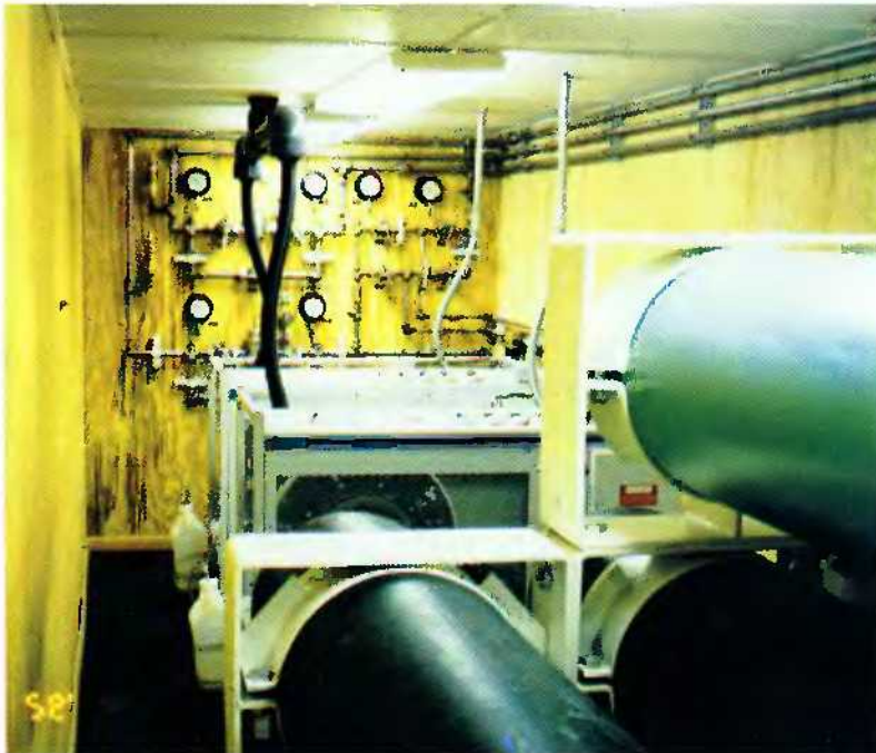
Pressure Adjustment room in 'sharm El-Sheikh
