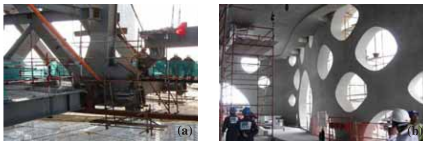
Figure (149) Detail showing the difference between Dia-grid construction case of steel and concrete, (a) Steel, (b) Concrete.
