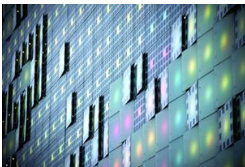
(Fig. 4.21) Some of the glass panels tilt outward, adding to the aesthetic effect of GreenPix.
