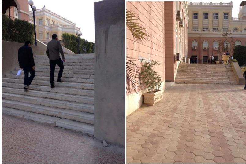
Fig. 91 BUE's broken steps that causes stumbling
