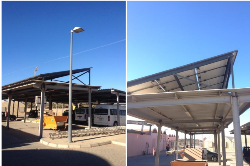
Fig. 154 PV cells used to generate electricity for lighting parking lots at RISE
