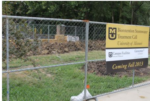
Fig. 14 The construction board of the project of the bioretention in Missouri (University of Missouri Campus Facilities, 2013)
