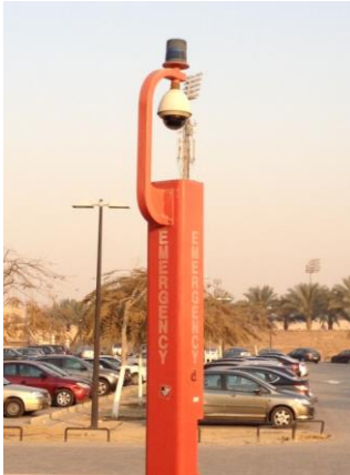
Fig. 151 Emergency call boxes and cameras
