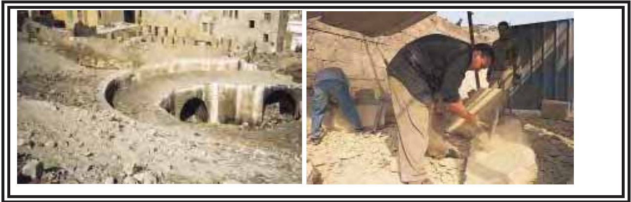
Figure 6-20 The most prominent tower of the Ayyubid wall (Bab al-Mahruq) still buried in debris (1994). A mason cutting stone for wall restoration
