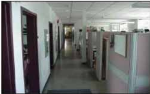
Hallway with no Electric Lighting
