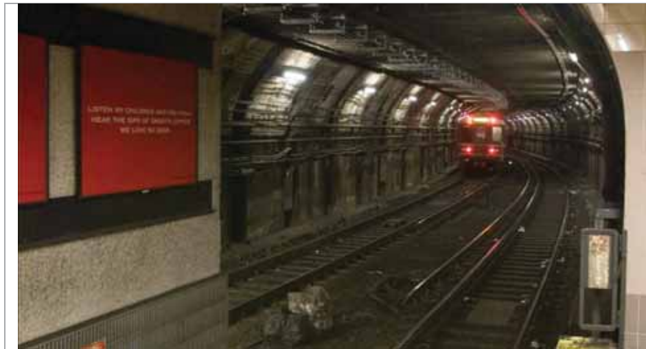
Figure 4-37: Spray-On Cementitious Treatment On Walls. MBTA Red Line Outbound Train Approaching South Station Viewed From Inbound Platform*
