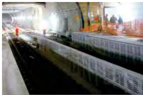
Figure 4-5: Platform And Noise-Absorbent Baffles Between Tracks And On Sidewalls Of The Under-Platform At Magenta Station Paris, France.‡
