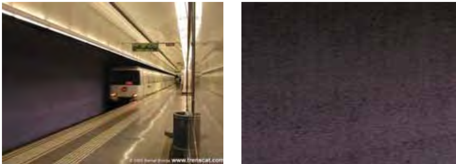
Figure 4-11: Spray-On Cementitious Sound Absorbing Material On Station Wall With Attractive Color And Texture. Barcelona Metro Line2 Tetuan Station.†
