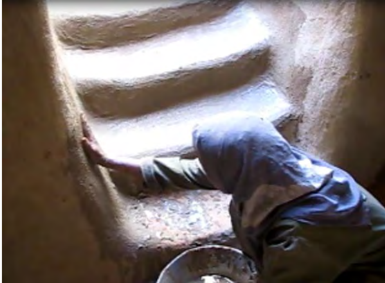
Figure 2.37 Monthly plastering maintenance for houses done regularly by women in the Dakhla oasis.
