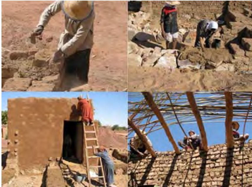
Figure 5.39 The built room of the neo-desert vernacular model house during different work phases.
