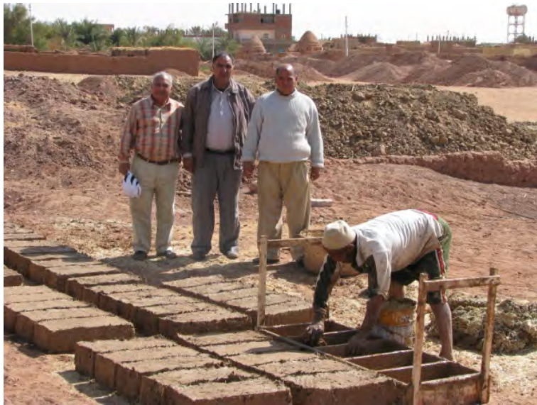
Figure 5.12 Mud brick casting using the first alternative of the mould and the representatives from the local municipality visiting the site to follow the work in process.
