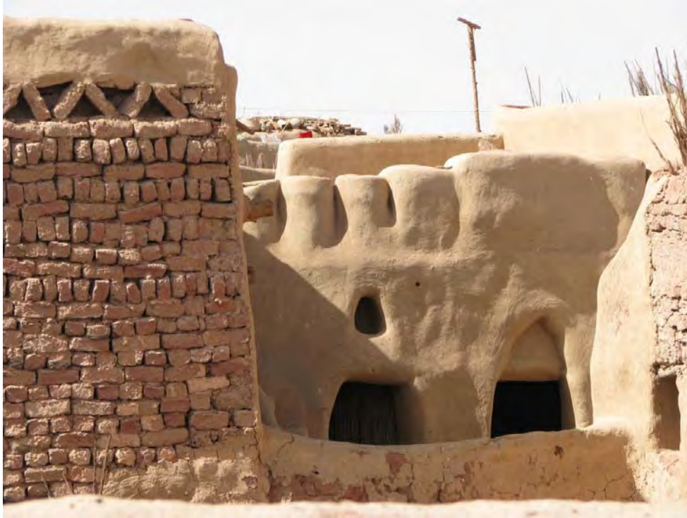
Figure 4.28 Parapets, openings and wheat storage are pieces of hand sculptures in Balat.
