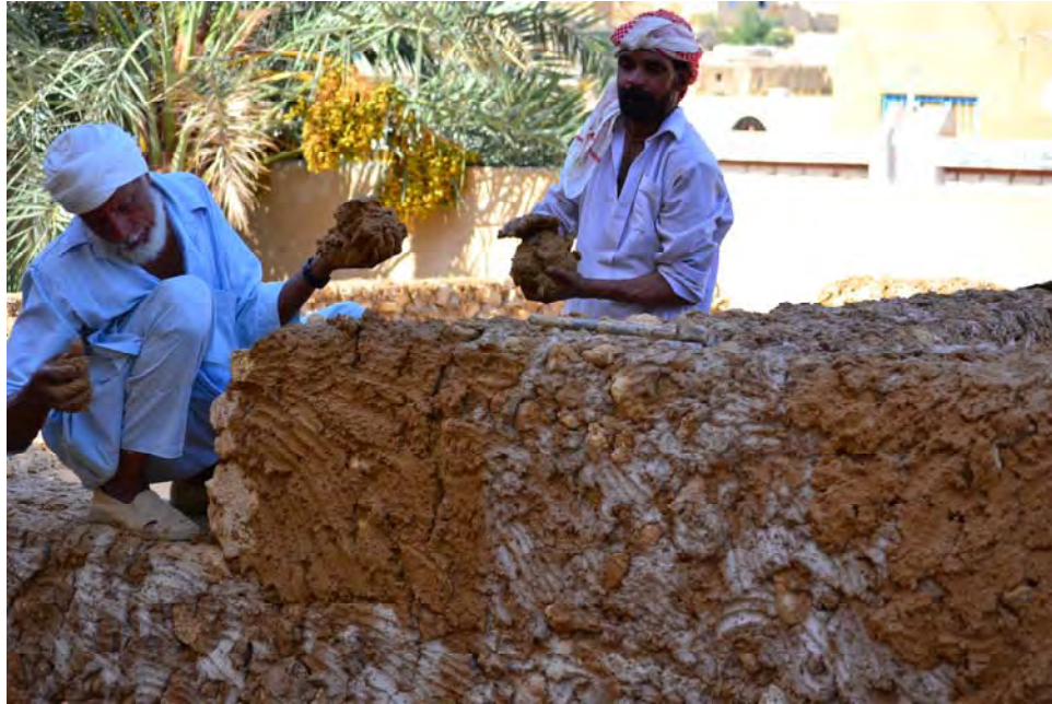
Figure 2.15 Vernacular builders in the Siwa oasis using salt blocks (Karshif) and mud. Roof construction is palm wood and mud brick.
