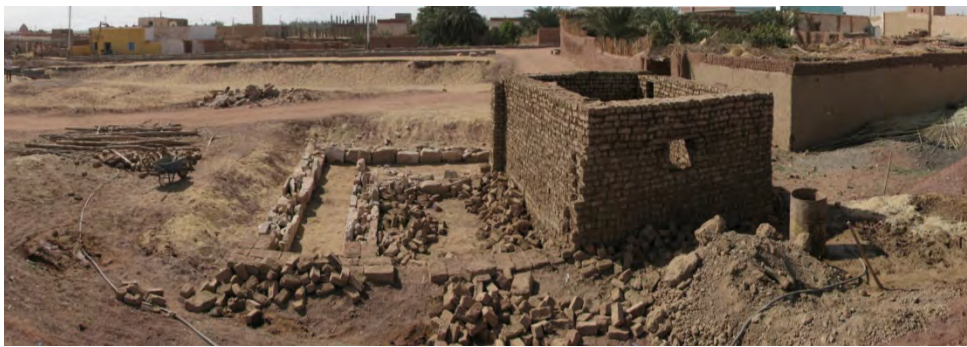
Figure 5.9 The site during construction for the neo-desert vernacular model, showing the foundation of the house and the room during construction.
