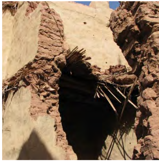
Figure 4.90 A part of a deteriorated house showing wall thickness made from mud bricks.
