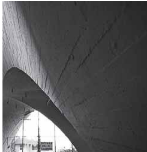
Fig. 1.50: Shape of the inner concrete surface. Source: Petra Gruber, Biomimetics in Architecture: Architecture of Life and Buildings , SpringerWienNewYork, 2011.
