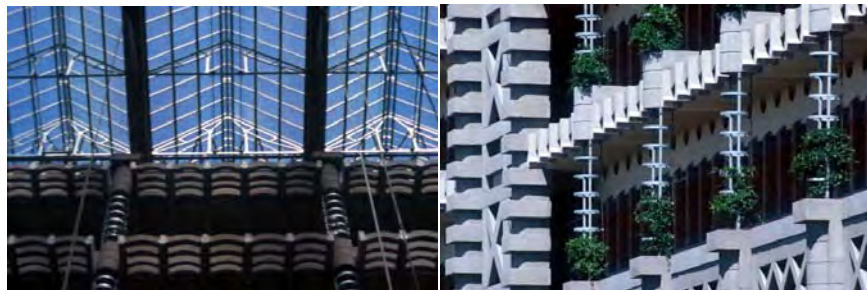
Figure (a-16) The Façade Shows the Exhaust Air Ducts. (Johnston, 2001)
