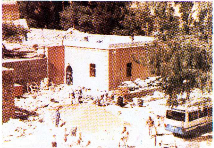
• A general view of the east resthouse outside the Monastery during restoration.
