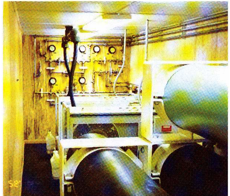
Pressure Adjustment room in sharm El-Sheikh
