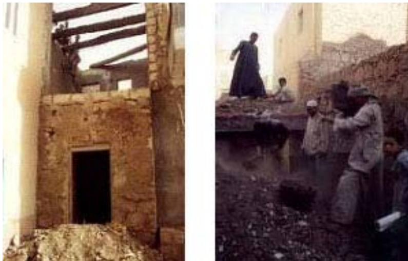
Figure 5. Roofless al-Sawada houses before upgrading & Neighbours join forces as upgrading begins, (Source: BLACD)
