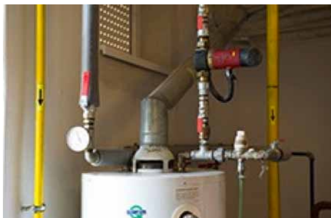
Heating system, Bratislava (EBRD)
