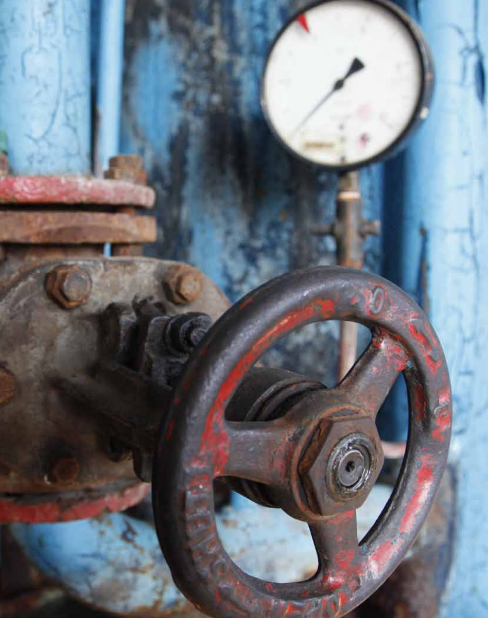
Energy efficiency retrofit of Moldava's largest producer and exporter of fruit juice and canned vegetables. EBRD financed.
