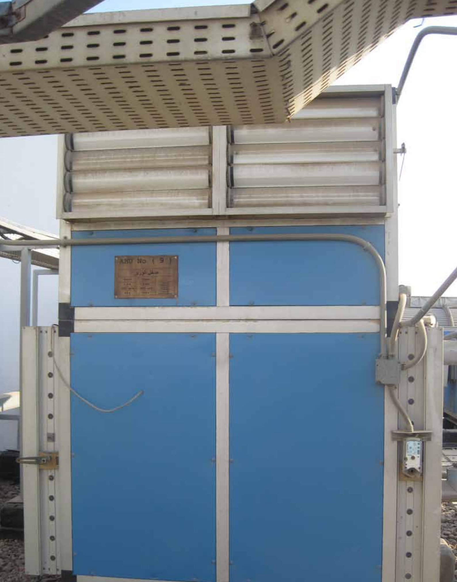
Energy efficiency HVAC system (Heating, Ventilation and Air Conditioning)
