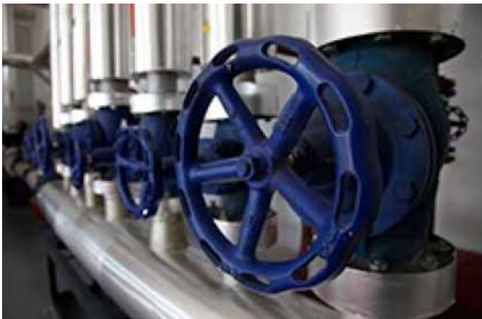
Energy efficiency retrofit of a heating system in a school building in Bratislava (EBRD)
