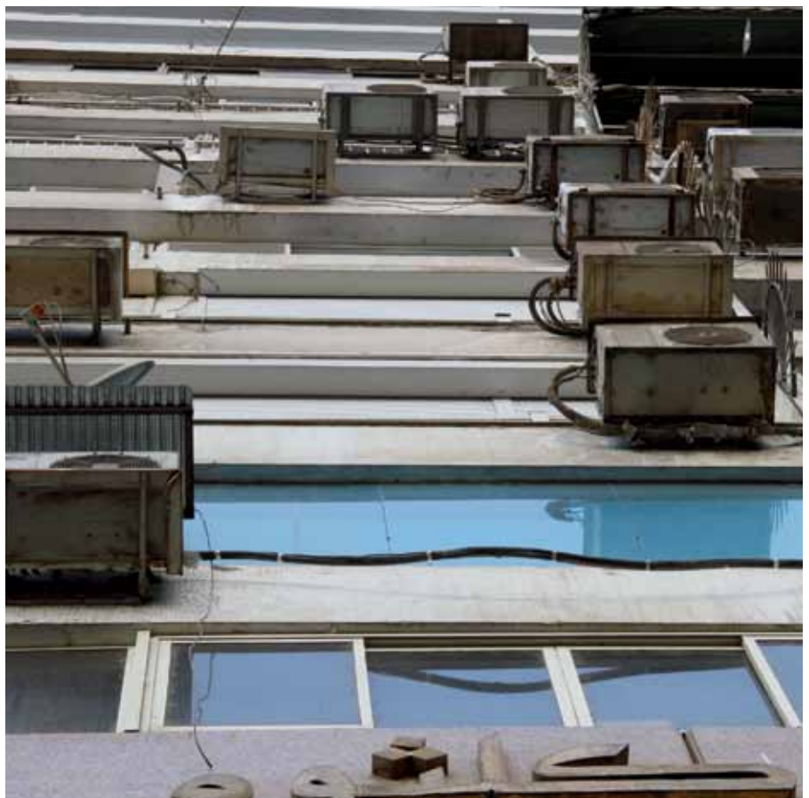
Low energy prices lead to inefficient use of resources – multiple old air conditioning units on a building in Egypt
