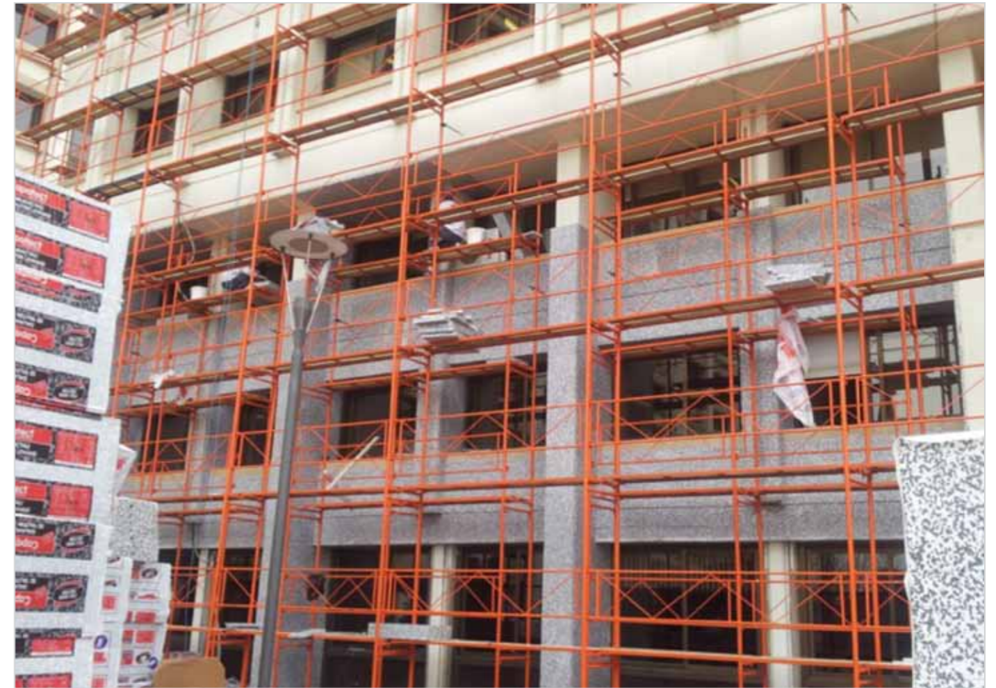
The government to set a good example: insulation work at the Turkish Ministry of Energy
