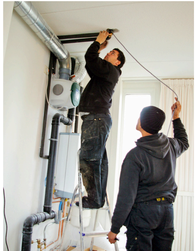
Renovation of heating and air conditioning systems can also radically improve the energy efficiency of existing buildings
